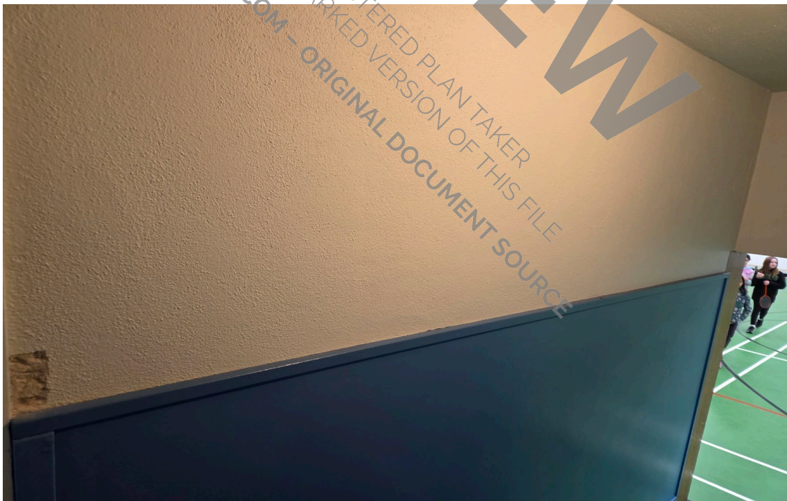
Photo 2: Location of east stairwell with asbestos containing skim coat/joint compound.
